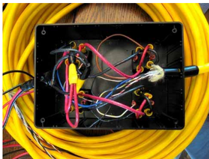
Figure 12: This is what the inside of the control box looked like before we added the camera wires.
