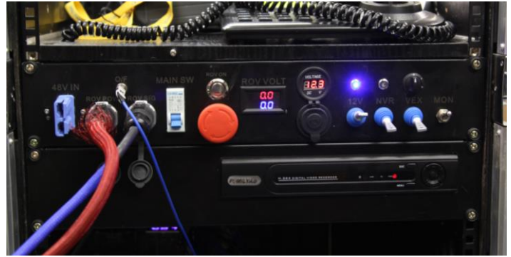
Figure 33: Front side of the Electrical Distribution Control Panel
